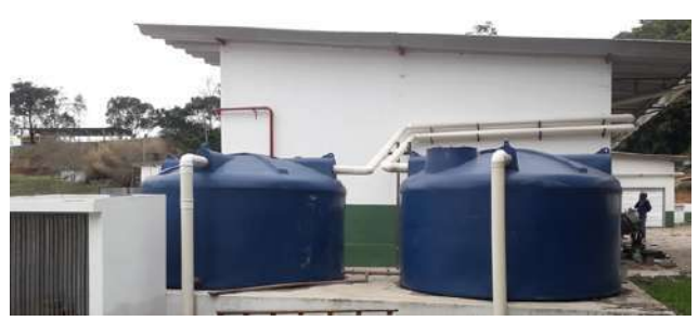
Figure 24: Carmo de Minas Campus water reservoirs connected to the rainwater collection system.
