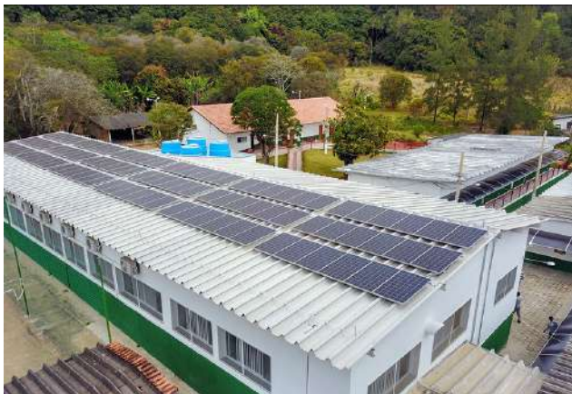
Figure 3: Carmo de Minas Campus photovoltaic panels for solar energy production through the IF Solar Program.
