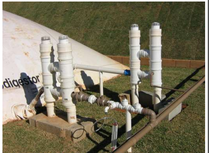
Figure 14. Swine waste treatment unit for biogas production.
