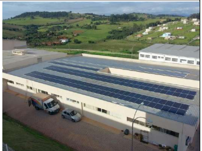
Figure 6: Campus Pouso Alegre solar power plant.
