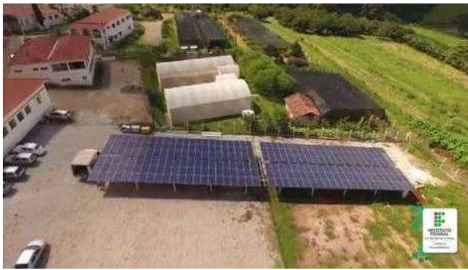
Figure 3: Campus Muzambinho solar power plant.
