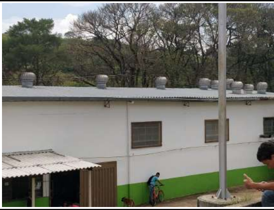
Figure 15: Campus Machado Coffee Roasting Building exhausters.
