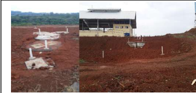
Figure 5: Muzambinho Campus waste treatment.
