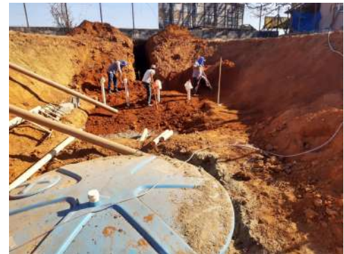
Figure 10: Machado Campus construction of Sewage Treatment Network in Center of Excellence of Coffee.
