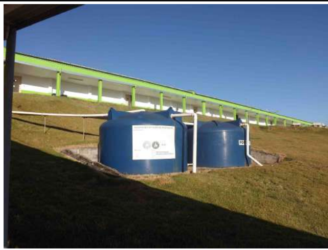
Figure 6: Machado Campus rainwater reservoir tanks.
