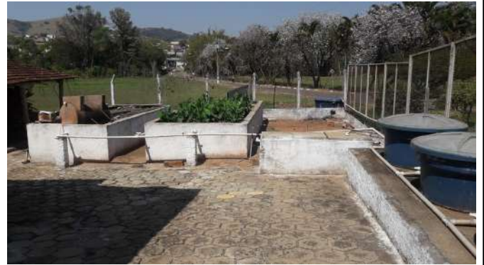
Figure 16: Inconfidentes Campus Wetland System installed in the dairy sector.
