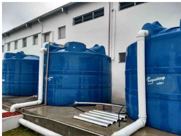
Figure 9: Poços de Caldas Campus rainwater reservoir tanks.
