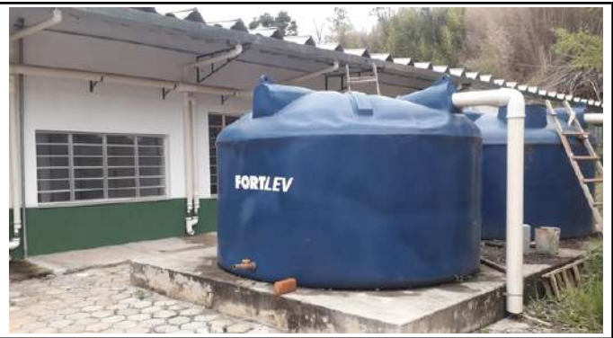
Figure 14: Carmo de Minas Campus rain harvesting system.
