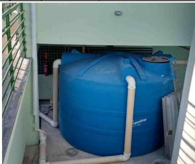
Figure 11: Rectory rainwater reservoir tank.
