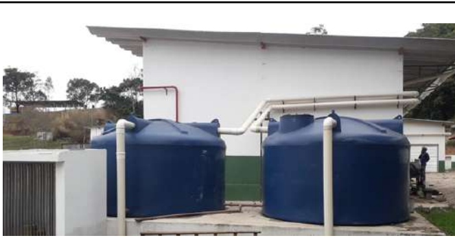
Figure 13: Carmo de Minas Campus rainwater reservoir tanks.
