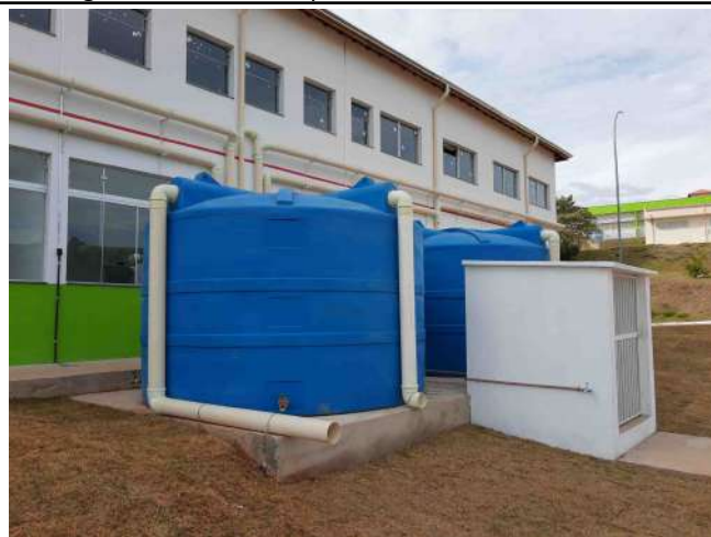
Figure 10: Pouso Alegre Campus rainwater reservoir tanks.
