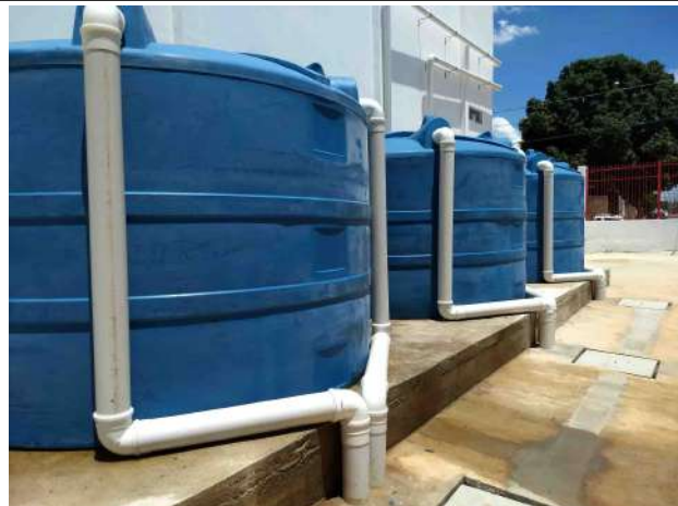
Figure 8: Passos Campus rainwater reservoir tanks.
