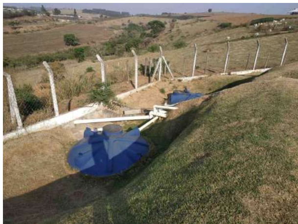
Figure 7: Muzambinho Campus rainwater reservoir tanks.
