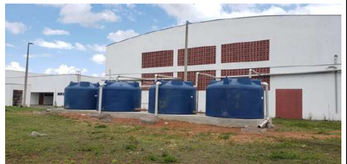
Figure 20: Poços de Caldas Campus rainwater reservoir tanks.
