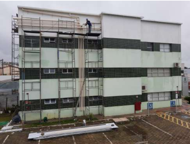
Figure 19: Rectory new rain harvesting system.
