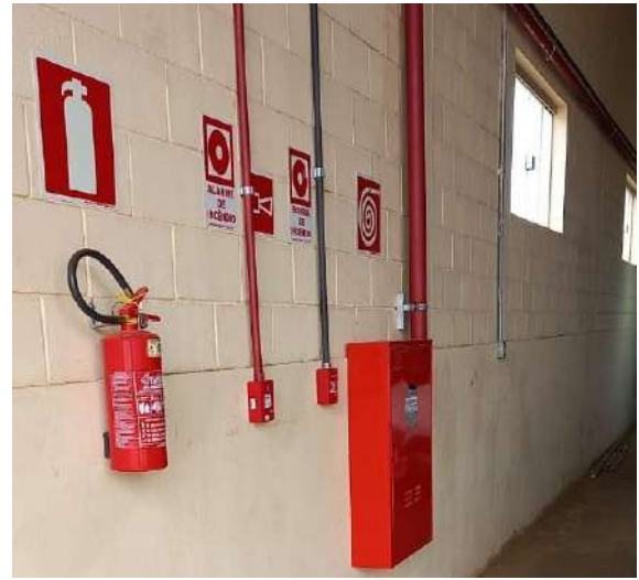
Figure 6: Pouso Alegre Campus fire alarm, fire extinguisher and hydrant.
