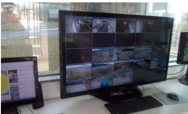
Figure 3: Machado Campus CCTV in entrance.
