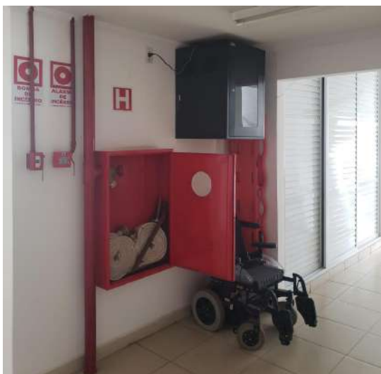
Figure 9: Rectory fire alarm and hydrant.
