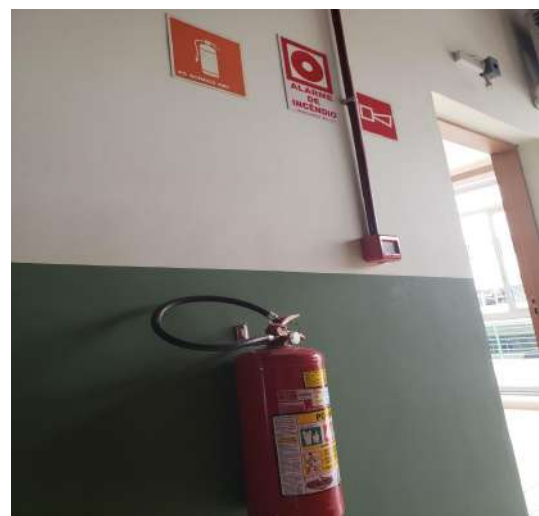
Figure 10: Rectory fire alarm and fire extinguisher.
