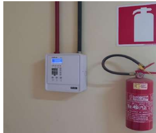
Figure 8: Pouso Alegre fire alarm and fire extinguisher.
