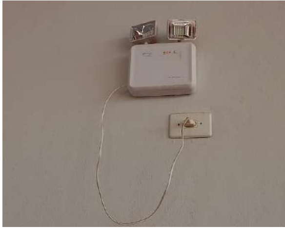
Figure 5: Pouso Alegre Campus emergency lights.
