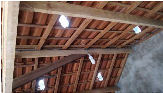
Figure 19: Inconfidentes Campus natural lighting with pet bottles filled with water.
