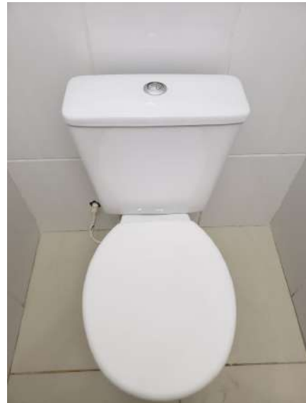
Figure 10: Rectory toilet flushing with double activation.
