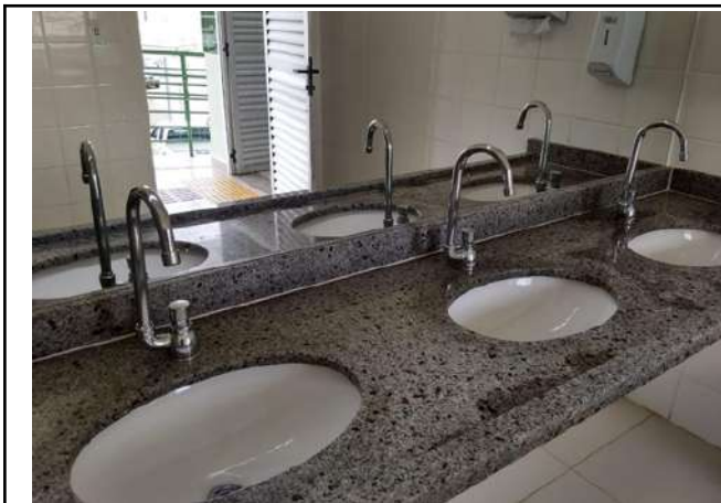
Figure 1: Rectory time delay water taps.
